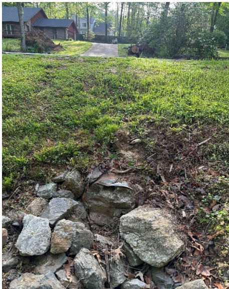
Photo of storm pipe with plug
